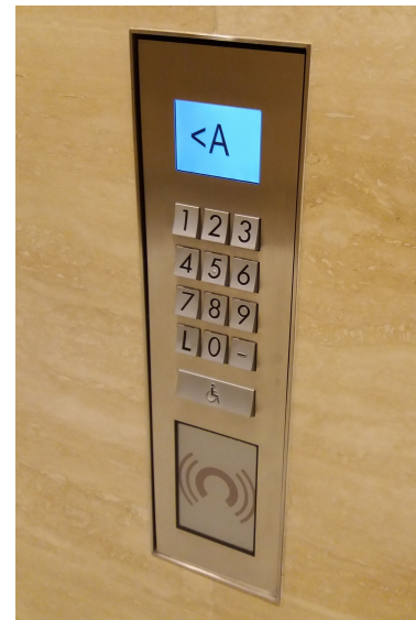
FIGURE 2.2: The numeric keypad used in destination dispatch control to enter the required destination floor. The passenger is assigned to elevator A in this case [45].
