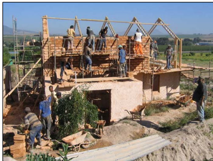
Figure 2: Builders working on one of the first buildings that form part of the Lynedoch EcoVillage project.
